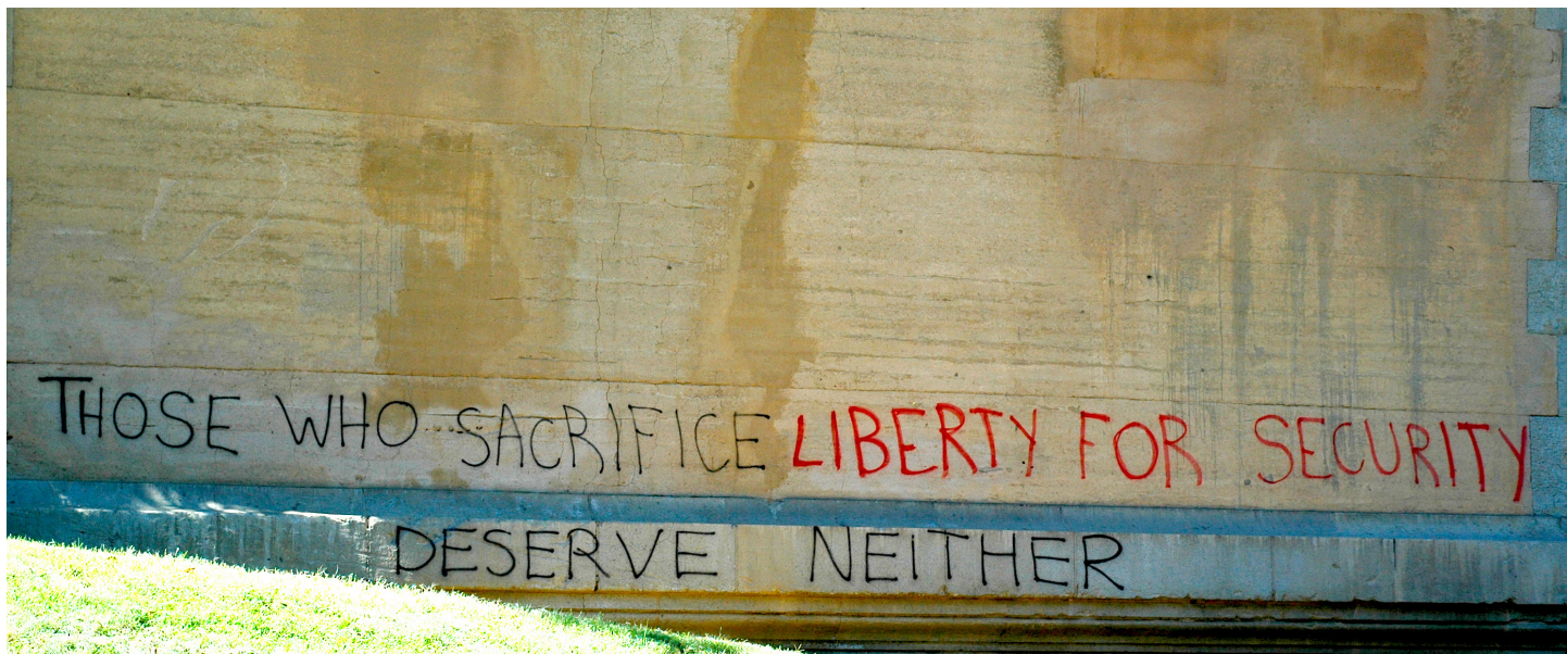
Graffiti on base of bridge in Rock Creek Park, Washington DC.
